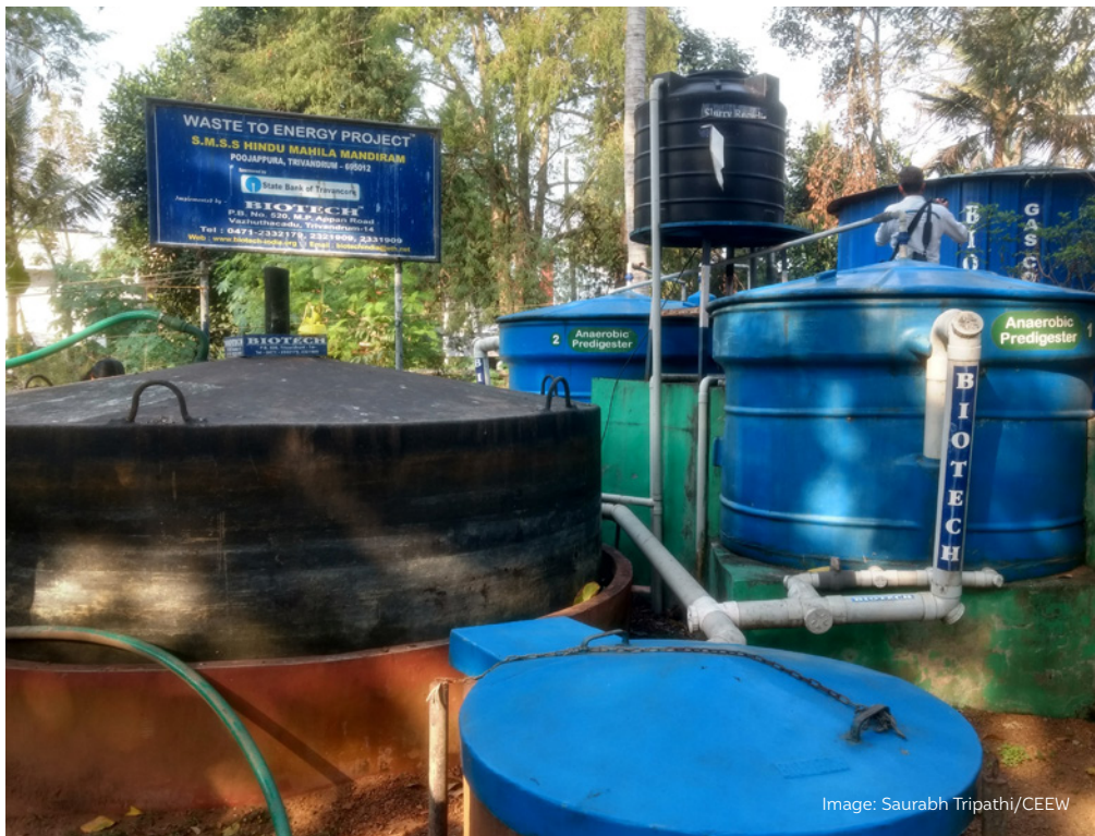
FIGURE 10: Community biogas plant
